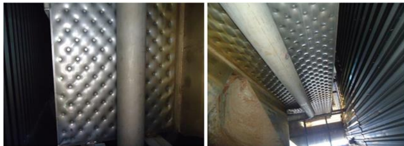
Figure 10: Heat exchanger inspection during plant outage after several months of real time biofilm monitoring.
